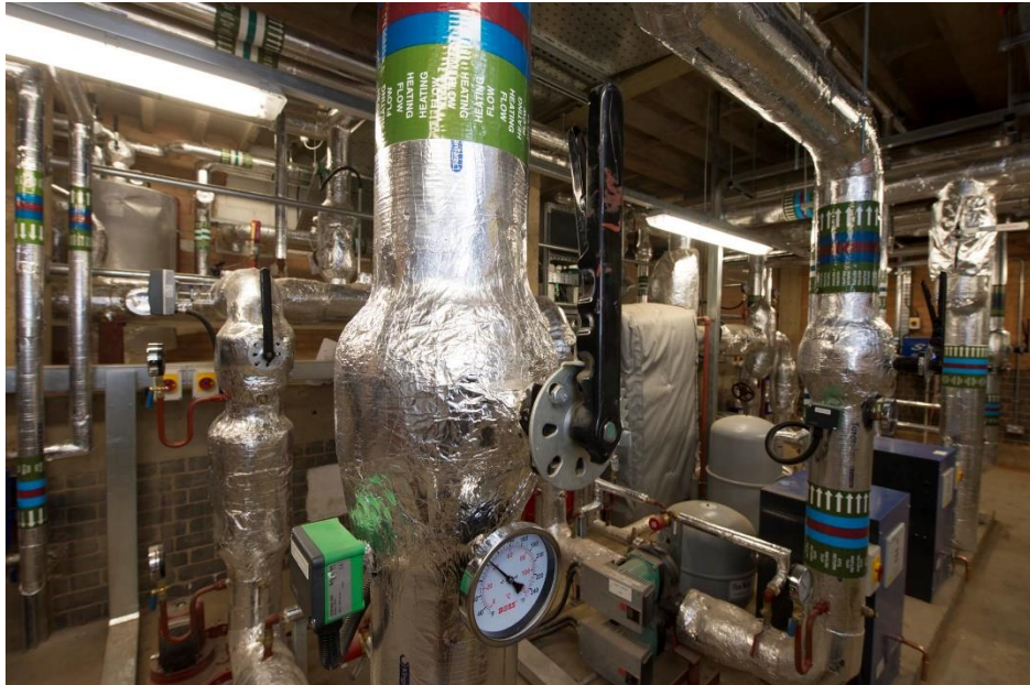
District heating, largest municipal network in UK
