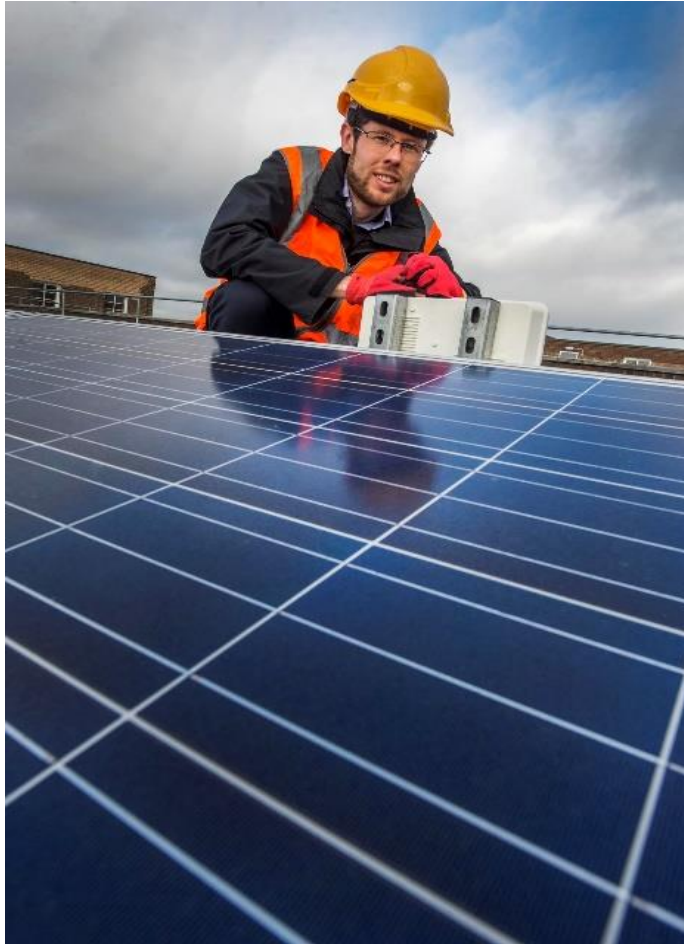
634 kWp PV systems on council buildings generating 524,954 kWh/y
